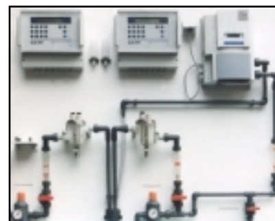
Drinking water quality panel waterworks Muldenberg
